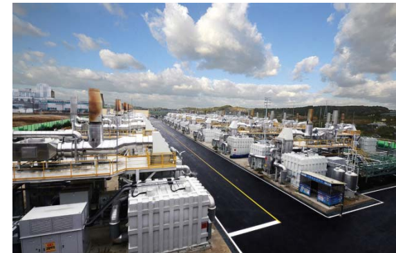
59-MW Gyeonggi Green Energy fuel cell park in Hwasung City, South Korea
