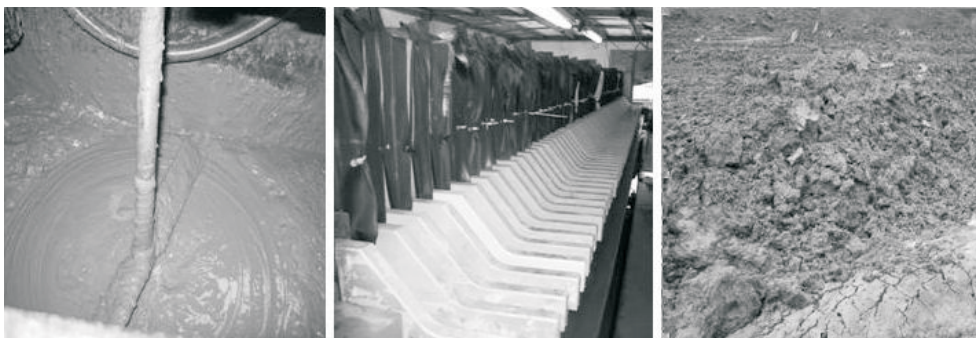
Fig. 1. Photo of used drilling mud, filtration press, and filtration cake destined for ground reclamation
